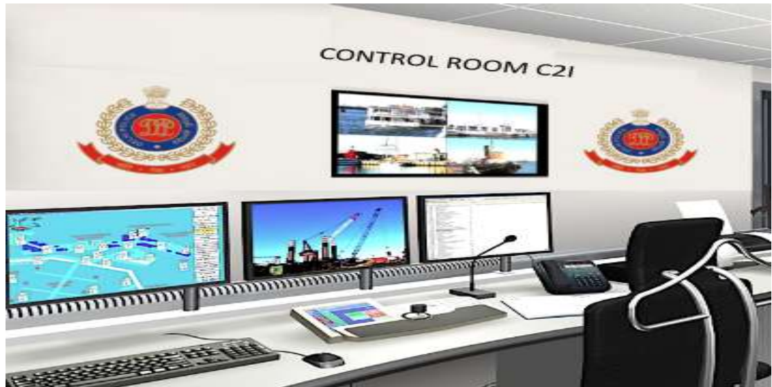
Figure: Control Room C2I – Single Seating Workstation
