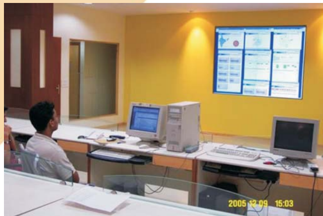
Grid Monitoring and Management Centre
