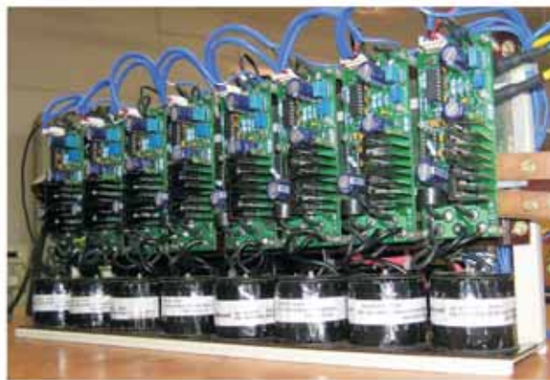
1 kW Fuel cell based power plant
