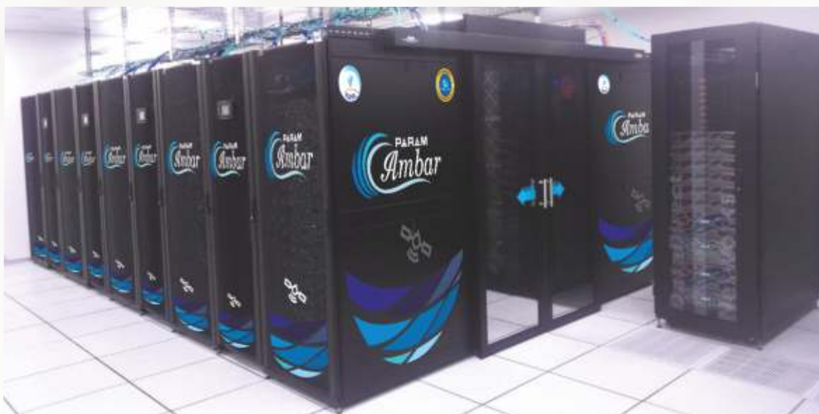
PARAM AMBAR Supercomputing facility at NARL
