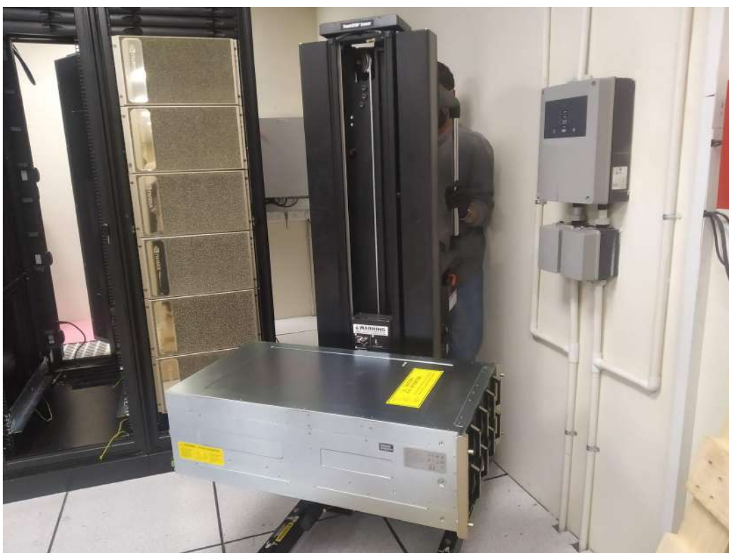
PARAM Siddhi-AI System Commissioning at NPSF, CIP.
