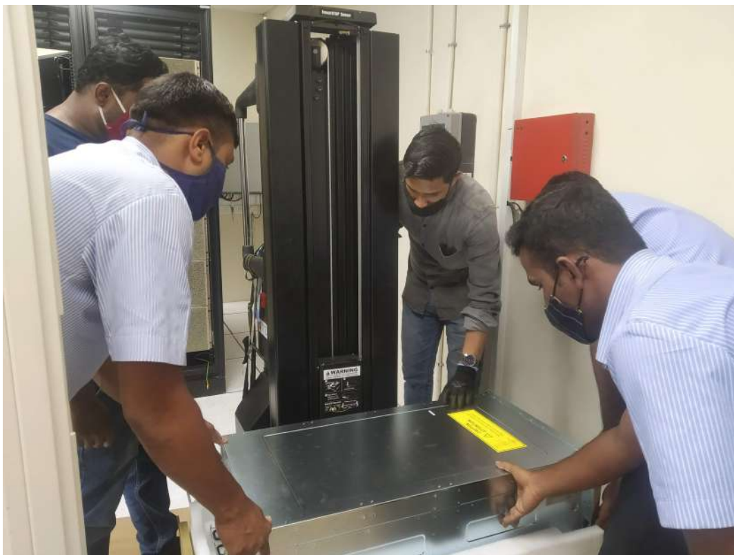
PARAM Siddhi-AI System Commissioning at NPSF, CIP.
