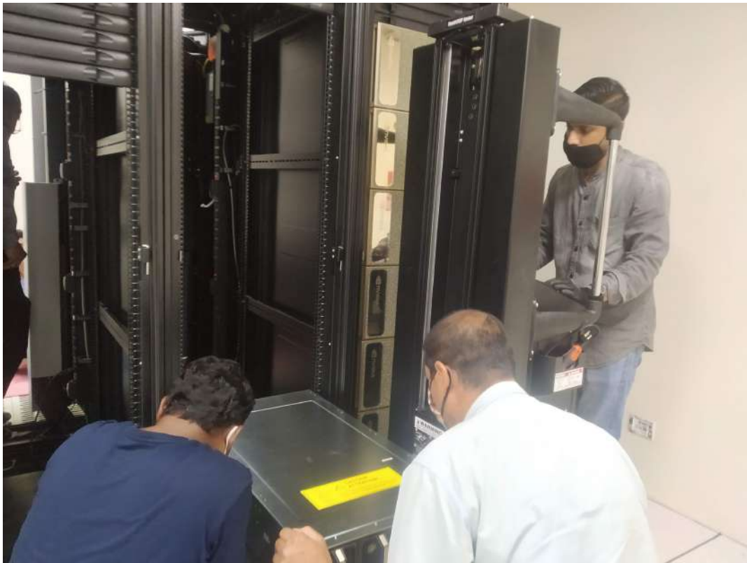
PARAM Siddhi-AI System Commissioning at NPSF, CIP.
