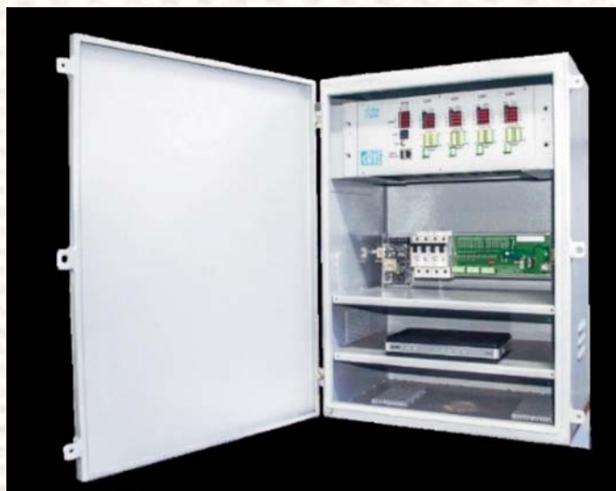
ACTSC System Installation
