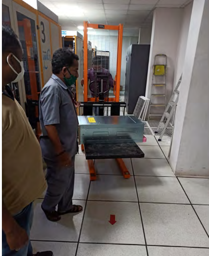
PARAM Siddhi-AI System Installation at NPSF
