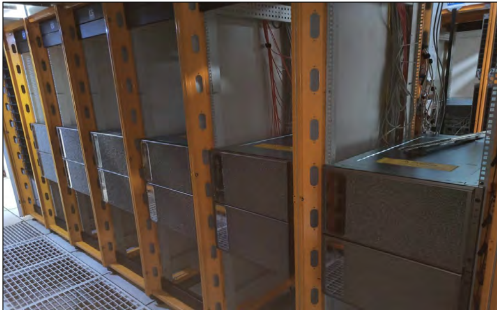
PARAM Siddhi-AI System Installation at NPSF
