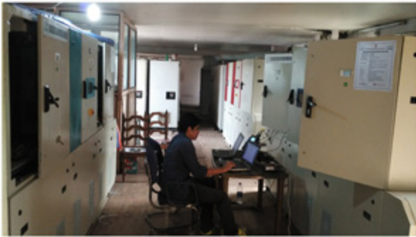
Installation at Jamuria, West Bengal
